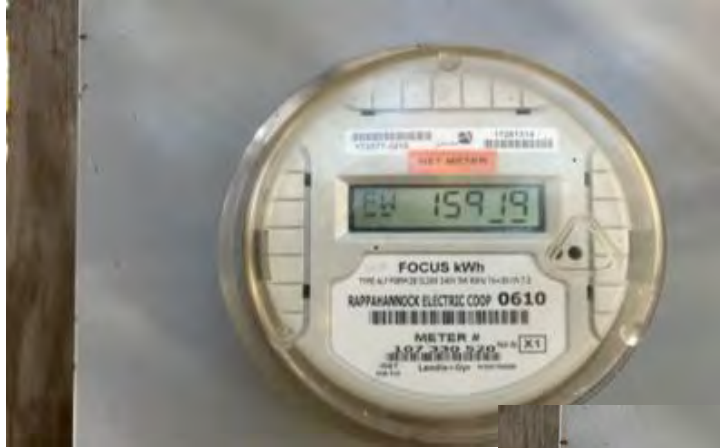
Forward Meter reading
