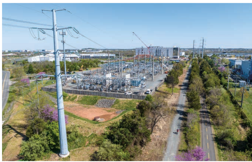
A substation being built next to the WO&D Trail. Photo by Hugh Kenny
