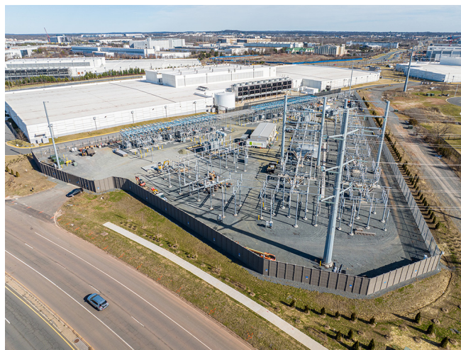
Data center in Loudoun County. Credit: Hugh Kenny, PEC.
