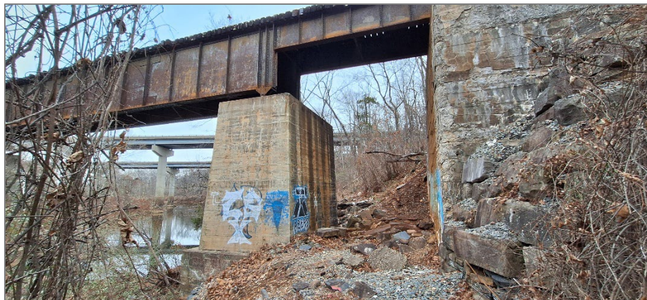
Vicinity of railroad trestle, showing need for trail construction, covered underpass shelter (approx. 70' length), bank stabilization/restoration, and general maintenance.
